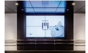
5 Toranomom Underground Passage Digital Signage
